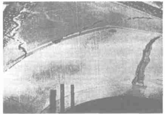
图 4 捷克古教堂因交通振动产生的裂缝 Fig. 4 Vibration induced crack of an old church near road
